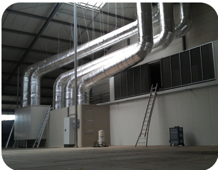
Industrial air scrubber
